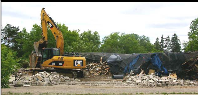
The recent demolition of Baden Sheet Metal on Brewery Street makes way for more development possibly.
